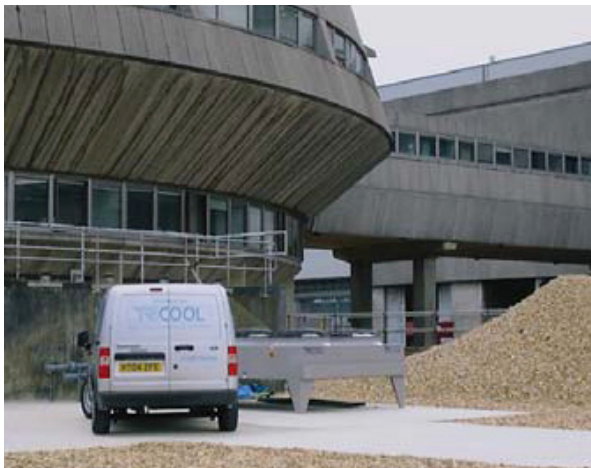
Tricool Thermal offer a cost-effective solution to Fawley power station
