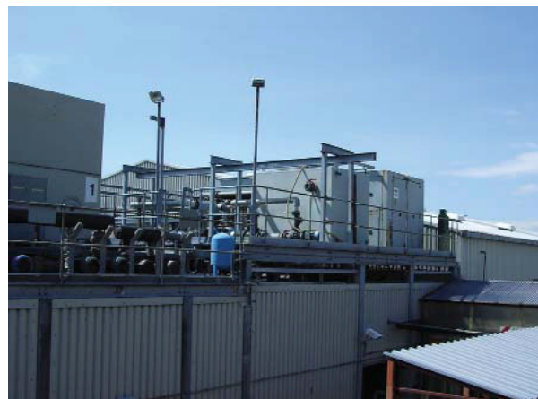
Tricool Thermal roof mounted cooling plant
