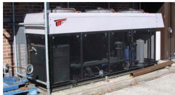
Fully weatherproof cooling package
