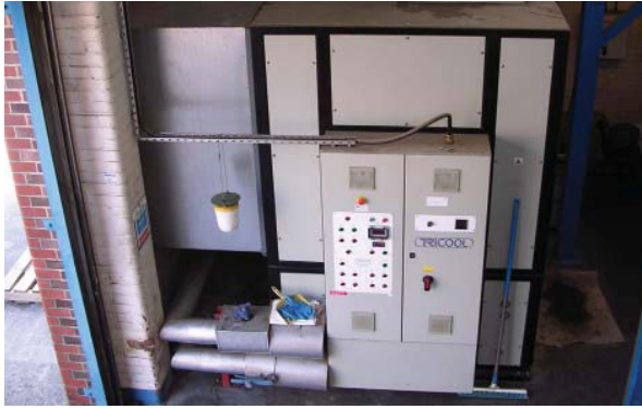
Internal localised controls for plant
