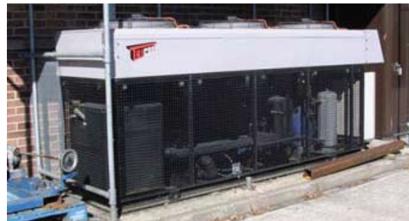
Fully weatherproof cooling package
