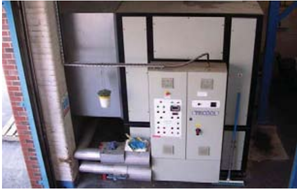
Internal localised controls for plant
