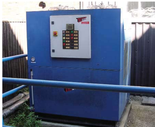
Tricool Thermal's cooling plant
