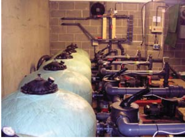
Tricool Thermal's purpose-built internal water circulation plant
